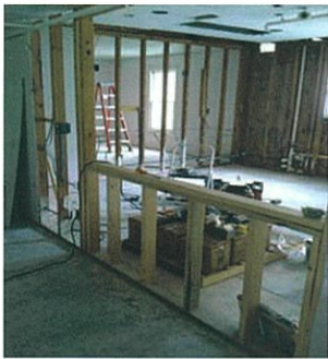
Kitchen before rehab
